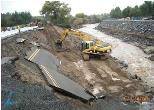
The storm of December 2010 caused serious damage to Mockingbird Canyon Road
