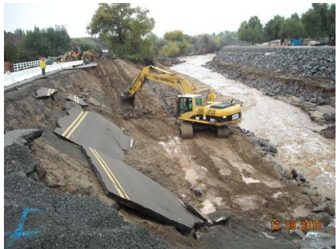
The storm of December 2010 caused serious damage to Mockingbird Canyon Road
